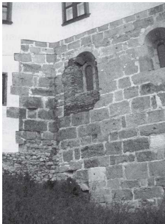
Fig. 7 - Ptuj Castle, corner joint between the southern wall of the 12 th -century hall and the perimeter wall (after SCHICHT 2010, Fig. 197).
